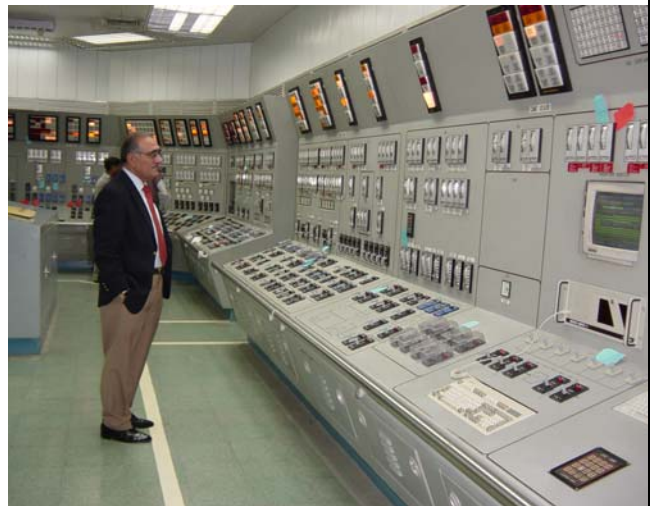
Figure 7. Author visiting CHASNUPP Control Room, November 2003
